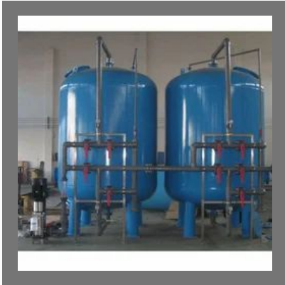
DM Water Plant
