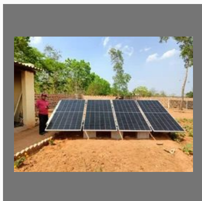
Off Grid Solar Power Plant set up
