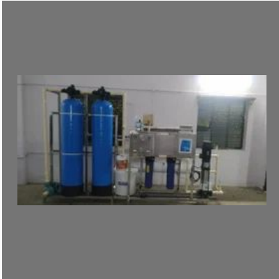
FRP RO Plant
