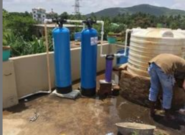
Water Treatment Plants
